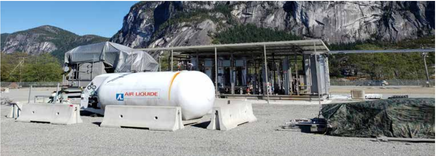
Carbon Engineering pilot plant in Squamish, B.C. (Photo credit: Tracey Saxby)
